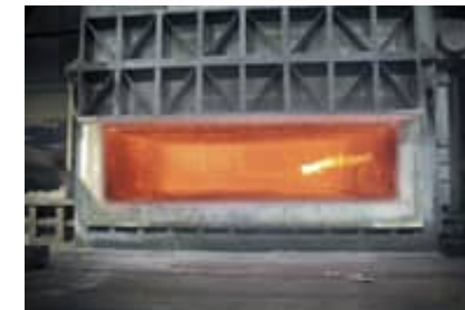
APPLICATION: Aluminum melting furnace
